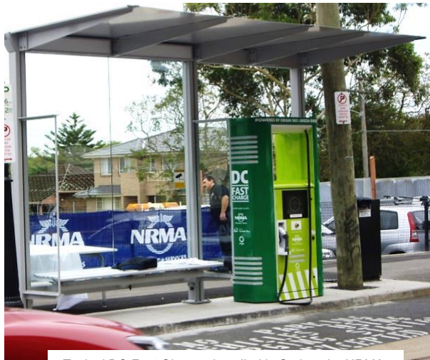
Typical DC Fast Charger installed in Sydney by NRMA Motoring Services
